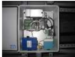
Vibrating wire and temperature sensors datalogger
