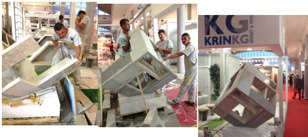
Figure, 8: Construction of the Box Packing structure of natural stone and the final installation at the Belgrade Stone Expo 2016
