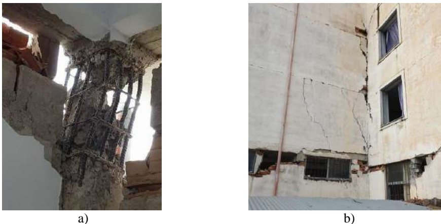
Figure 2 – Damage of a school building in Maminas, Albania: a) failure of the RC column and b) damaged masonry infill walls [6]
