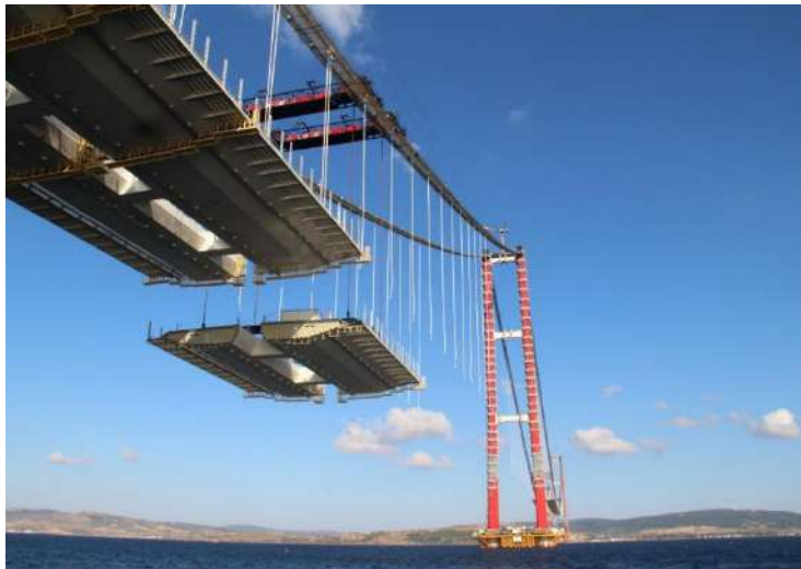
Figure 7 – Erection of deck segments using lifting gantries operating on top of the main cables.
