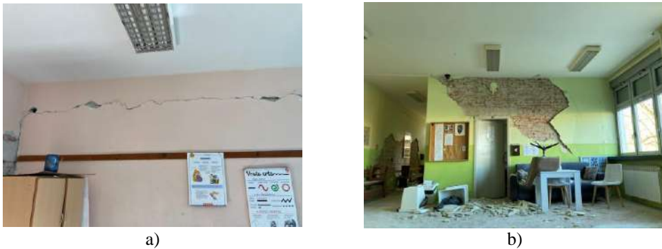
Figure 4 – Damage of RC schools in Petrinja, Croatia: a) cracks at the infill-frame interface, school Dragutin Tadijanović and b) damage of infill walls and plaster spalling, the Faculty of Education
