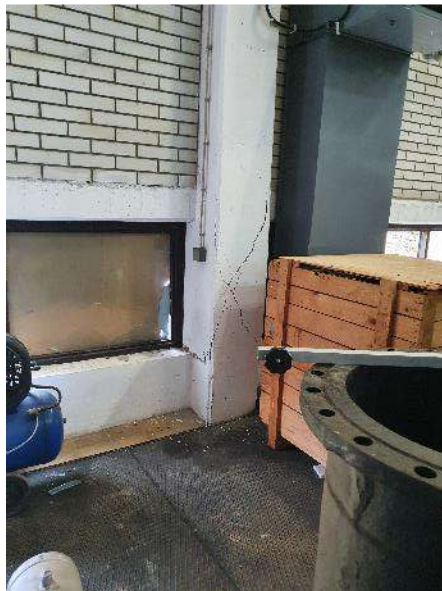
Figure 6 – View of one diagonal crack
