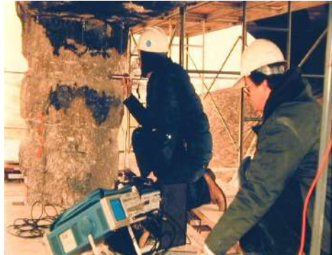
Figure 15 - Fire damaged concrete pier
