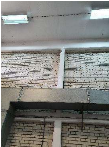
Figure 7 – Out of plane displacement of the westward masonry wall
