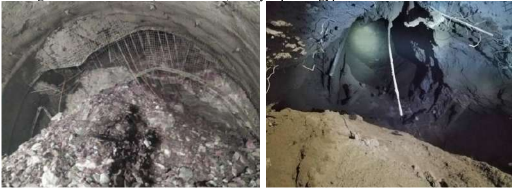
Figure 10 – Loss of stability at the occurrence of cavern in the roof of the right tube of tunnel Ivan
